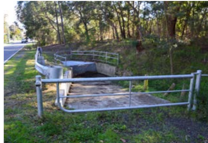
Galvanised Stainless Steel Stormwater Fence and Gates
