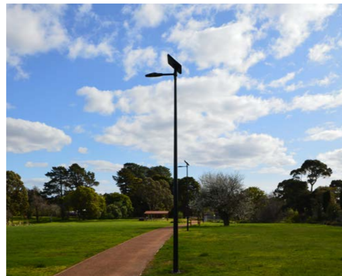
Solar powered path lighting, ngarrak nakorang wilam park Source: AECOM
